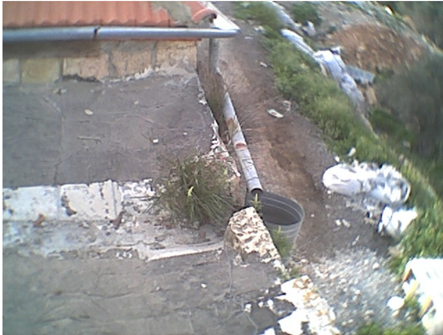
Photo 3.5.3: First-flush diverter (Ramallah).
