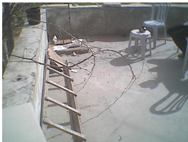
Photo 3.7.1.3: Contamination due to poor maintenance and because catchments very closed to cistern (Abu Shekheidim).
